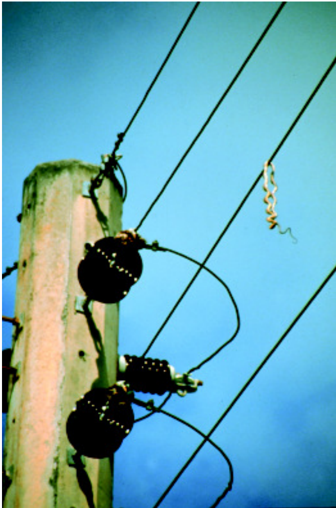
Each year on Guam, brown treesnakes cause many electrical power outages.
